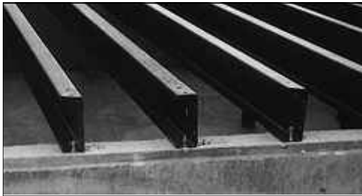
C or Z sectional steel joists bolted into position for first story flooring.
