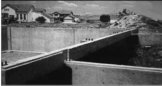
Foundation shows anchor bolt settings, and notched for panels. (Foundation By Others)
