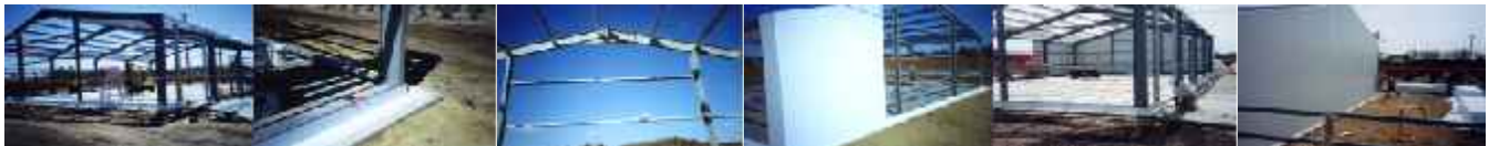
Tie Rods and all the bolts are tightened and checked to put building square.
